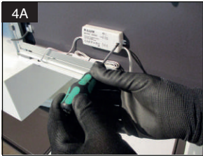
Open the infrared (IR) switch box (C)
